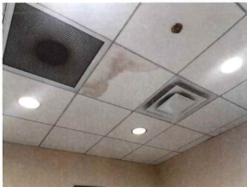
Replace ceiling tiles at water damage.
