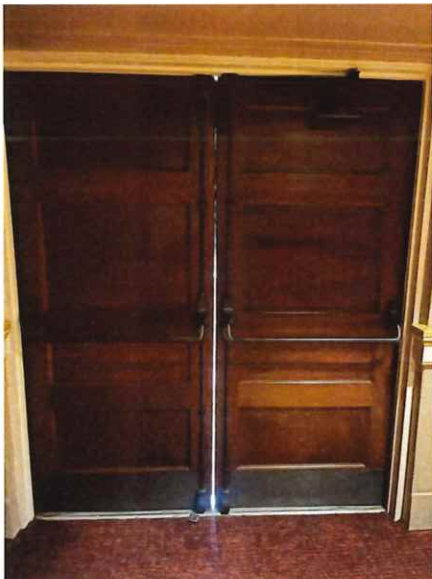
Weatherstripping to be replaced.
