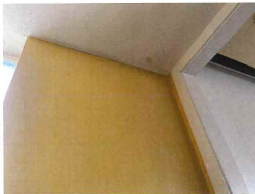
Ceiling damage, requires repainting.
