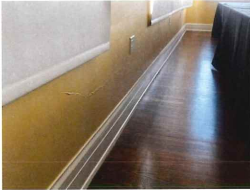
Bullock Ballroom wall damage at west wall.
