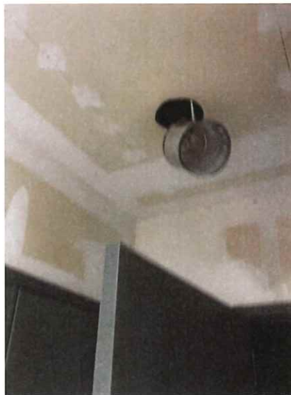
Fixture to be replaced at 3 rd floor.
