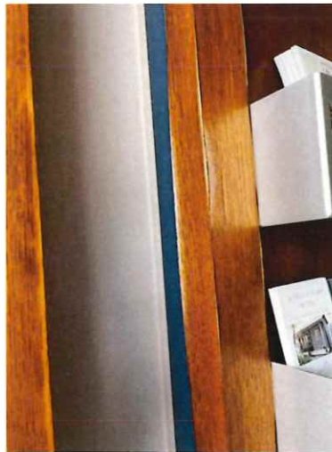
Millwork veneer is delaminating.
