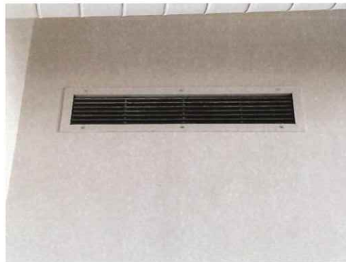
Clean registers. Ensure filters are changed.
